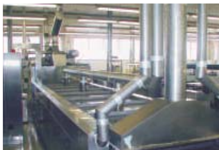
Industrial vessels and storage tanks
